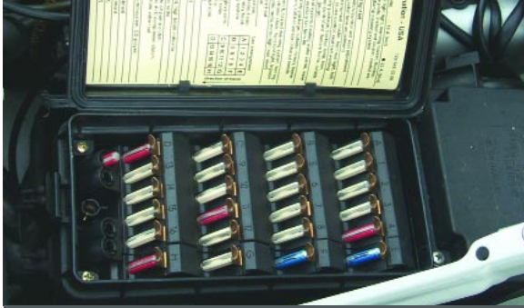
The fuse and relay box for most Mercedes-Benz cars is on the driver's side in the engine compartment, sealed with spring clips. Fuses and relays are clearly identified by position and number; voltage and continuity measurements are convenient.
